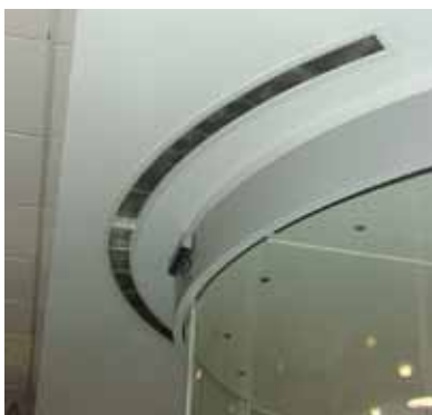
The discharge grille is precisely in line with the curve of the revolving door.
